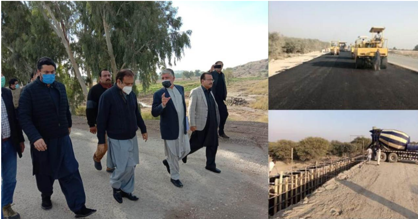
Federal Minister for Information & Broadcasting Senator Shibli Faraz and Chairman Kashmir Committee Shehryar Khan Afridi visiting under construction Pindi Gheb - Jand - Kohat Highway.
